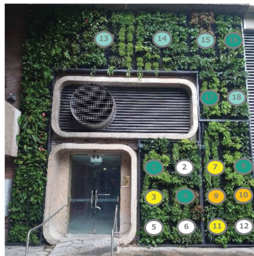
PHOTO COURTESY OF NTT LIMITED AND UNIVERSITY OF TECHNOLOGY SYDNEY RADIO FREQUENCY AND COMMUNICATION TECHNOLOGIES
