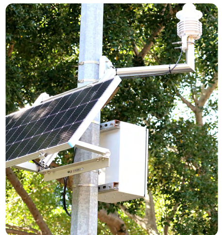
Environmental data is collected using weather stations installed throughout the park, to inform the SIMPaCT models that generate irrigation commands.
