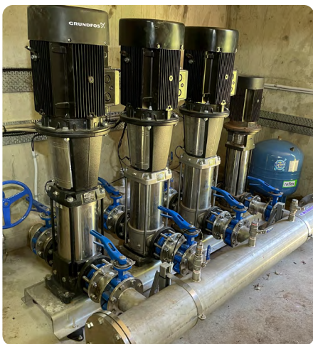
The pumps deliver recycled water across the diverse landscape of the park.
